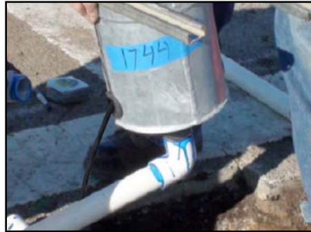
Base Can Attached to Drain Conduit
